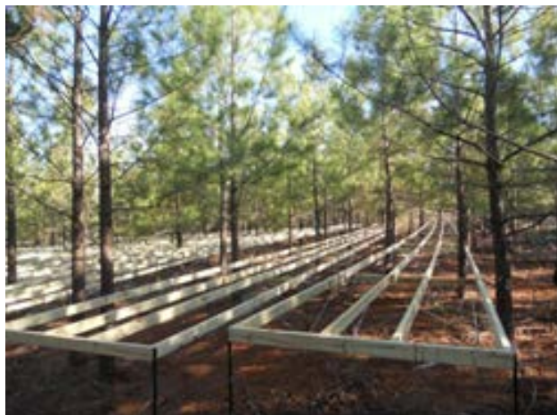
Figure 1b. Rain throughfall exclusion structures under construction at Tier III site in Buckingham County, Virginia. Photo courtesy of Tom Fox.
